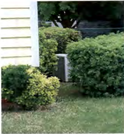
Utilities shielded from view with hedges.
