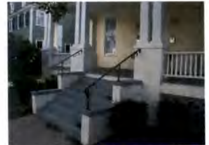
The metal stair railing was added to this porch stair as a safety feature. The use of a simple metal design does not detract from the historic porch and identifies it as a later addition.
