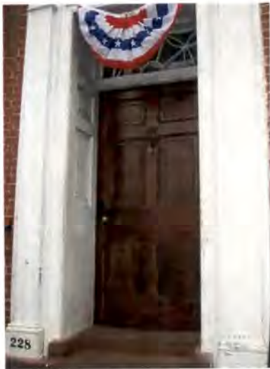
An example of a historic wood door that has been appropriately repaired instead of replaced.
